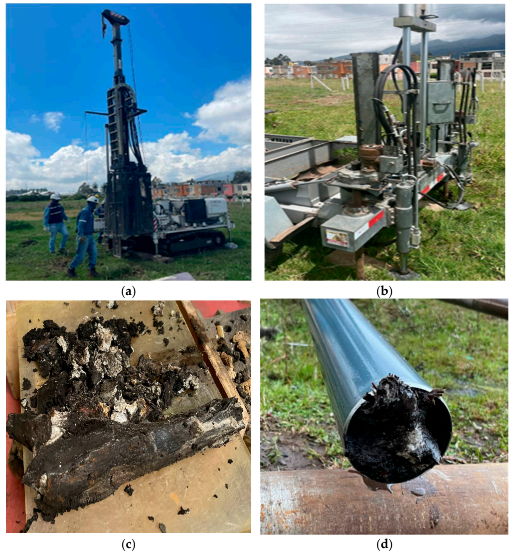
Figure 2. (a) Long Year drilling platform, (b) DMT platform, (c) wooden body found in a Shelby tube, and (d) mud found after Shelby's extraction.
