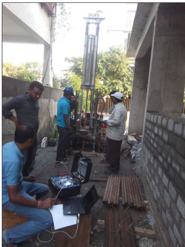
Fig. 6 Photograph showing test set up at Rajarhat test location
