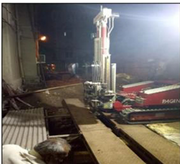
Fig. 3 Photograph showing test set up at High Court test location
